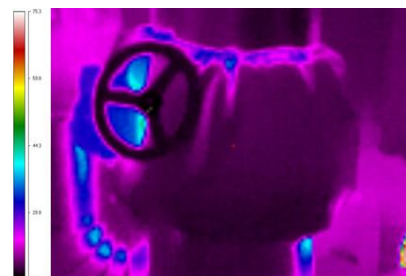
AFTER: insulation covers installed in 8 plant rooms. Surface temp 16C. Annual savings estimated at 500,000kWh, payback 1.4 years, 119 tonnesCO 2 e/year saved
