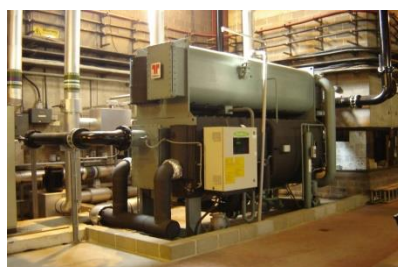
Our district chilled water via absorption chilling from waste heat
