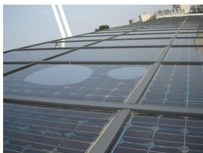
The 34kW photovoltaic system on the ZICER building
